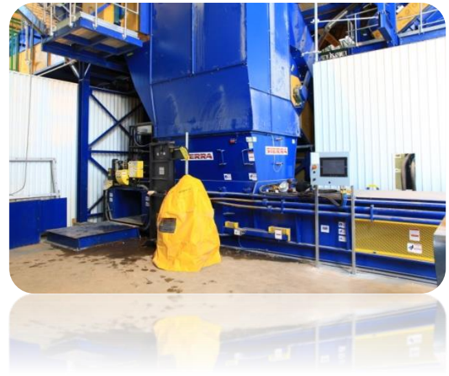
Dual Ram baler used to bale rejects and recyclables
