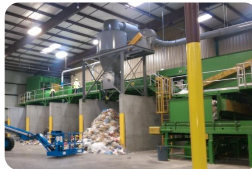
Air Vacuum System
